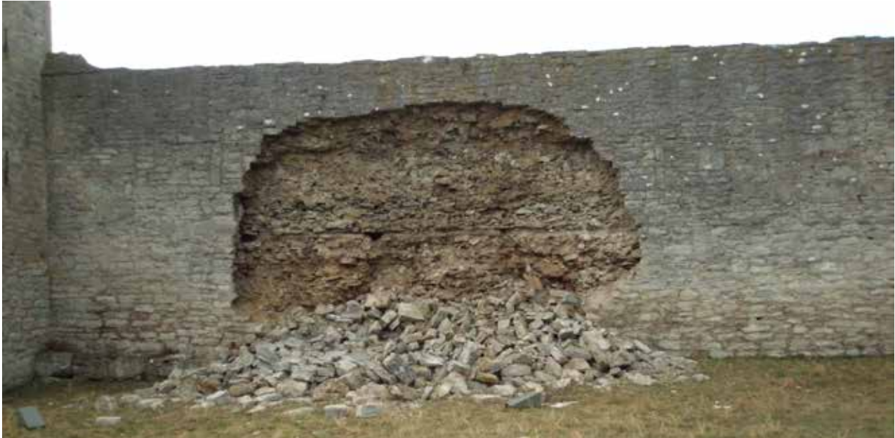
An example of a wall which was repointed with a sand-rich, non-elastic mortar.
