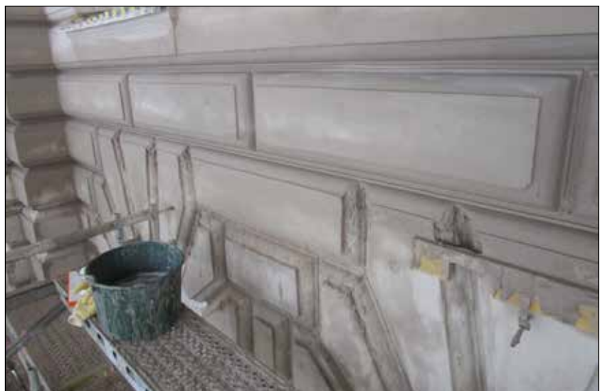
Template moulding in lime render. Photo: Simon Patetsos, TP Mur & Puts AB
