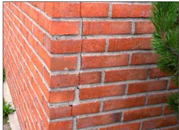
An example of a brick cavity wall expanding over the corners as a result of the horizontal joints forming long pressure bars.
